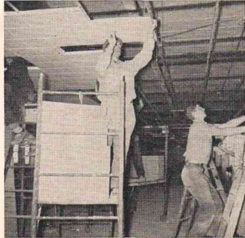
Workmen installing acoustical tiles at the new C.H.Q. The two-foot space between the floor above and the ceiling contains utilities and is easily accessible for repairs by the removal of one or more tiles.
